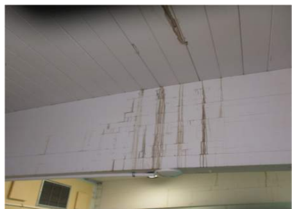
Typical Water Staining on Glulam Beam/Purlin and T&G Decking
