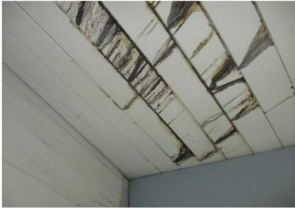
Water Staining at Western Ridge Beam End
