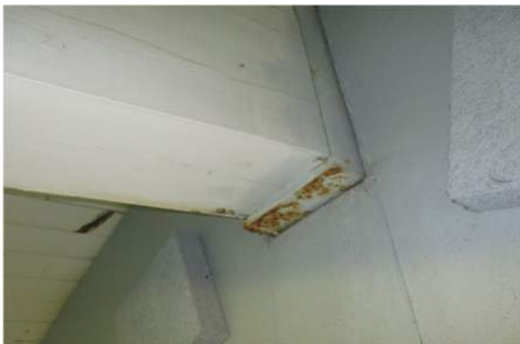
Superficial Rusting on Ridge Beam Hanger at West Wall
