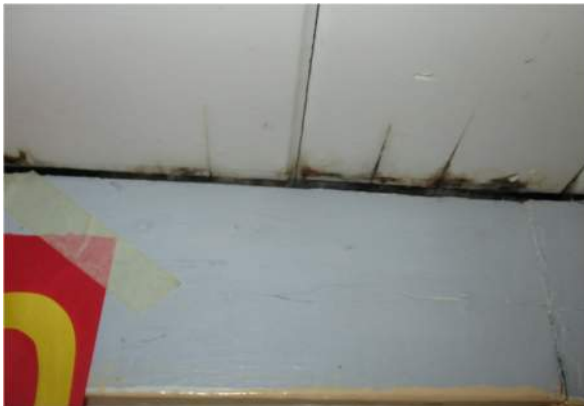
T&G Decking Water Staining at Eastern Wall
