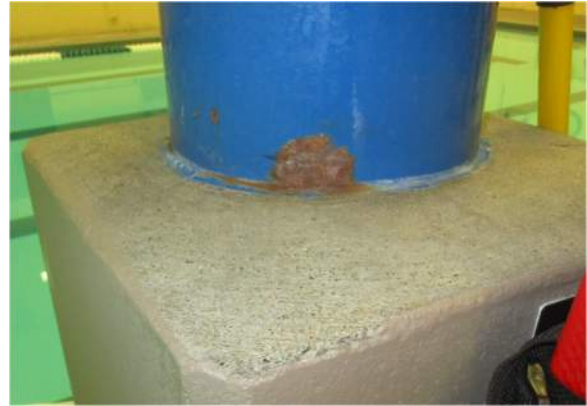
Rust at Base of 8" \varnothing Pipe Column
