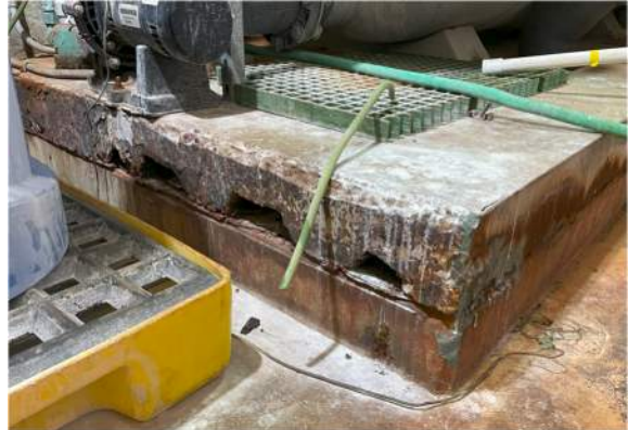
Pool Room Equipment Pad with Corroded Metal Deck and Spalling Slab
