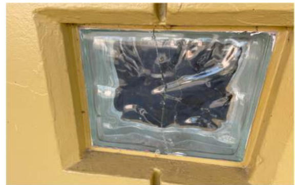
Cracked Glass Block Window at Eastern Wall
