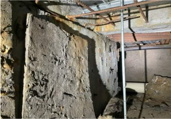
Exposed Rebar in Northwest Ventilation Tunnel
