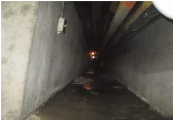
Mechanical Room Ventilation Tunnel Looking Northeast
