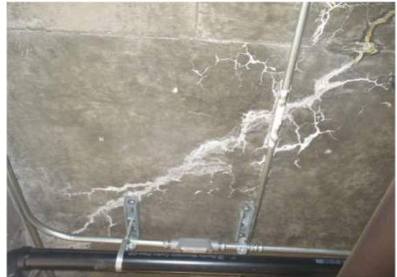
Cracking in Mechanical Room Ceiling Below Men's Locker Room
