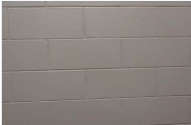
Minor Stair-step Mortar Crack in Men's Locker Room CMU Wall
