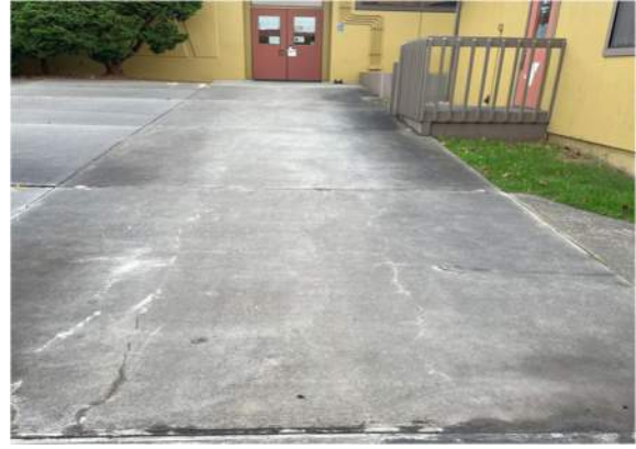
Cracking in Slab Above Mechanical Room Ventilation Tunnel
