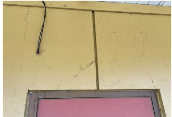
Temperature Cracking over Northeast Exit Door (Exterior)
