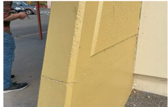
Cracking at Northwest Corner of Pool Building
