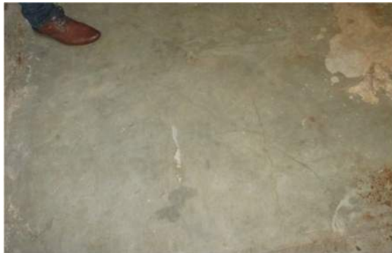
Minor Crack in Men's Locker Room Floor Slab
